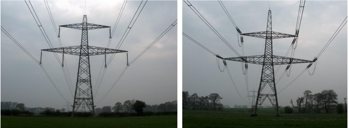
Image 4.17 Typical low height lattice pylon (suspension (left) and tension pylon (right)) 25
