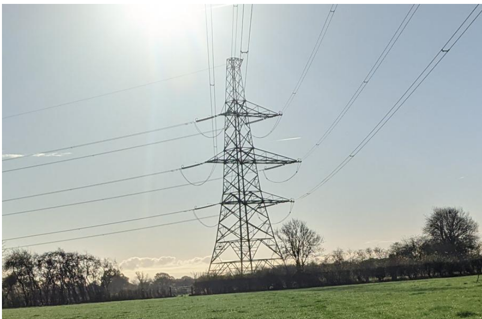
Image 4.16 Typical tension/angle lattice pylon 25
