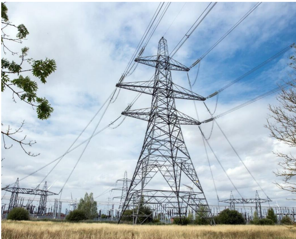
Image 4.18 Typical terminal lattice pylon 25
